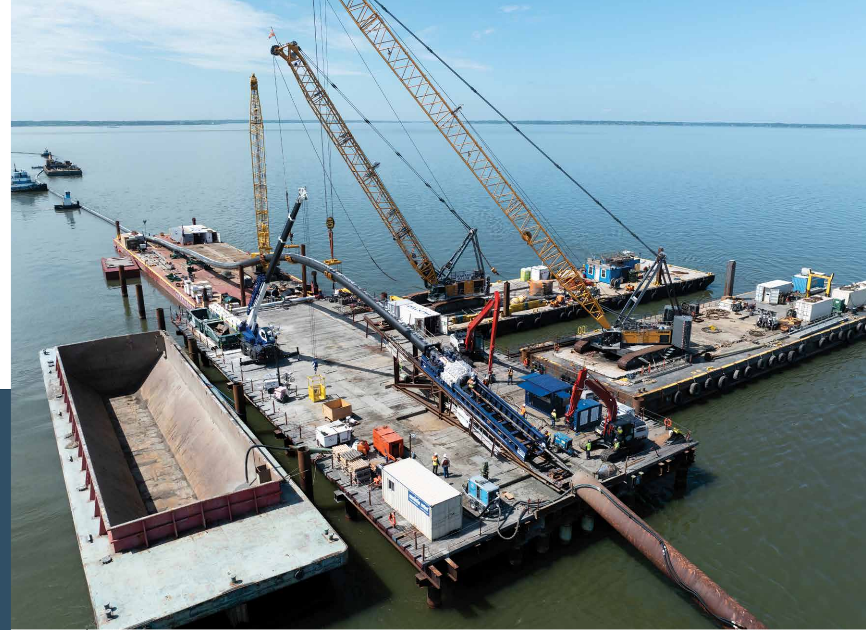
The Garney/Dewberry team completed a record breaking horizontal directional drill (HDD) under the Newport News shipping channel as part of our $145-million JRX project. Photo courtesy of Garney Construction.
